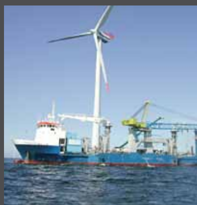
The Lincs Wind Farm, sponsored by Centrica Renewable Energy and two other joint-venture partners, is a proposed 270 MW wind farm being
